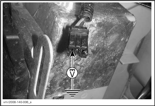
TAILLIGHT/BRAKE LIGHT INPUT VOLTAGE TEST
