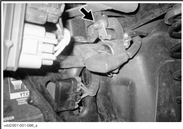
ELECTRICAL SYSTEM MAIN GROUND
